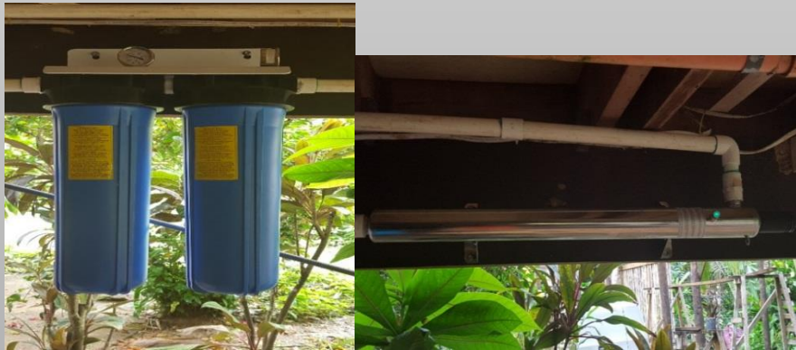
Our water filtration and UV treatment system
